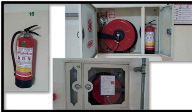
Picture 5: Fire Extinguishers and Fire Cabinets
