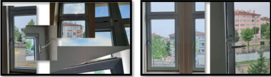
Picture 7: Window Locks
