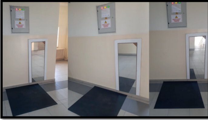
Picture 6: Electrical Panels and Insulator Mats
