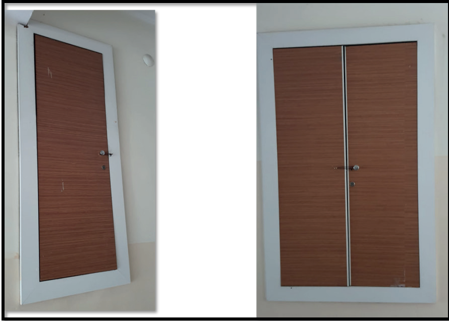
Picture 15: Locked Vent Covers
