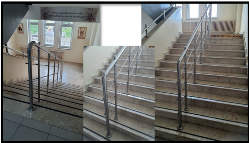
Picture 9: Handrails and Tapes
