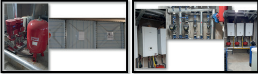
Picture 17: Water Tank and Combi Boiler Room
