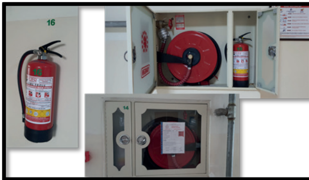
Picture 5: Fire Extinguishers and Fire Cabinets
