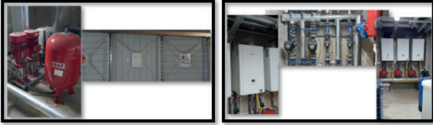
Picture 17: Water Tank and Combi Boiler Room
