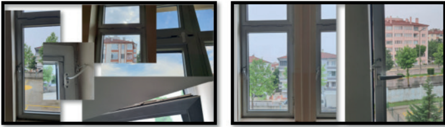
Picture 7: Window Locks
