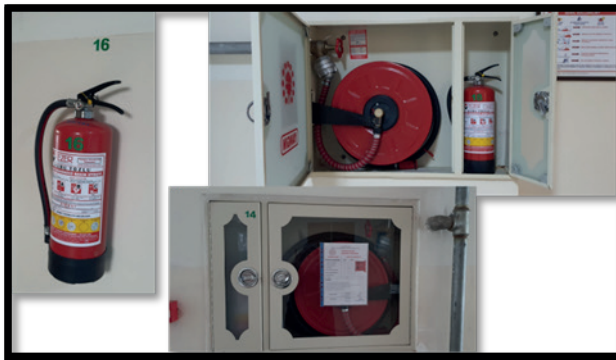
Picture 5: Fire Extinguishers and Fire Cabinets
