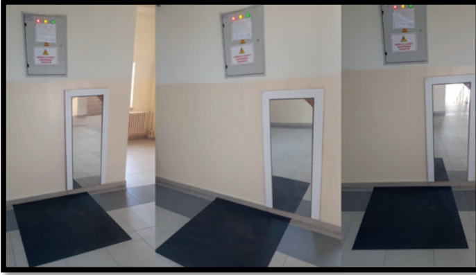
Picture 6: Electrical Panels and Insulator Mats
