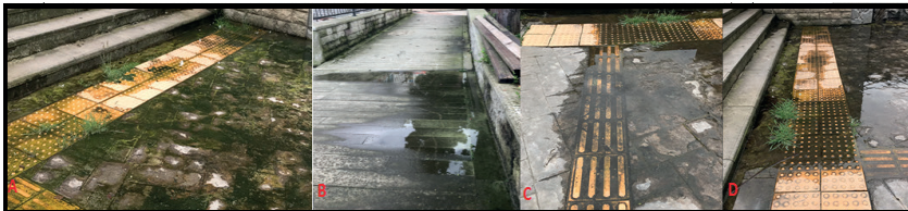
Figure 5. Water Accumulation, Eutrophication-Algae Growth, and Slipping Risk on Walkways Due to Faulty Drainage
