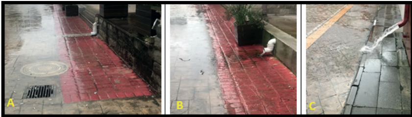
Figure 4. Discharge of Roof Water onto Pedestrian or Walkways
