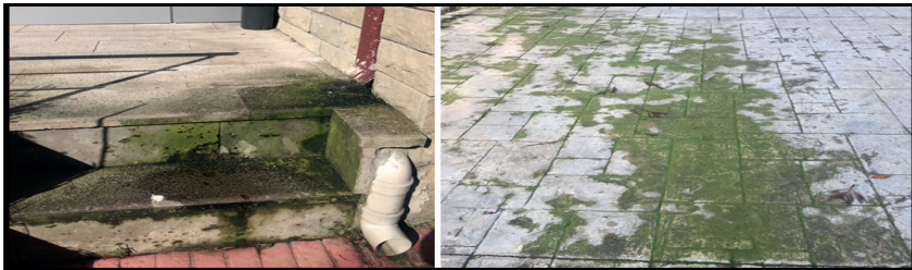
Figure 7. Slippery Conditions Caused by Algae Growth on Hard Surfaces Due to Rainwater
