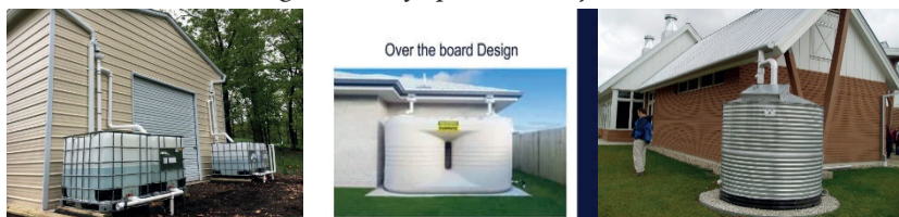
Figure 6. Rooftop collection systems
